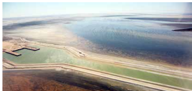
* The Cargo Transportation Route (CaTRo): Construction of the marine channel and control fill of the turning basin completed in August 2017
